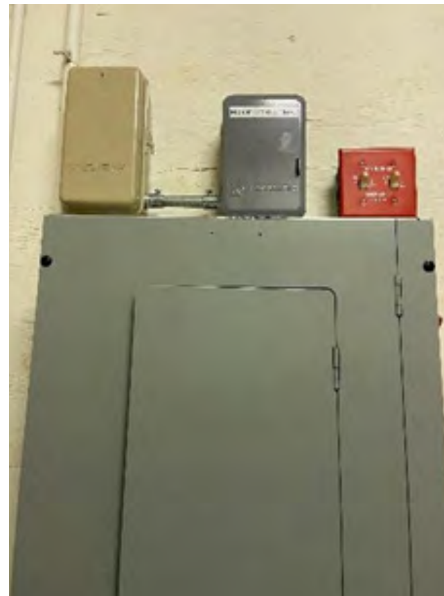
Newer Electrical Panel
