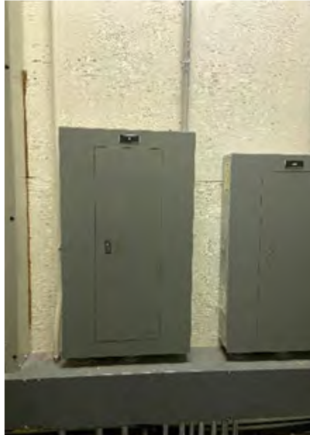
Older Electrical Panels
