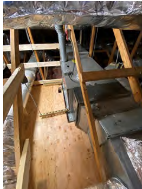
Furnace Unit in Attic Space
