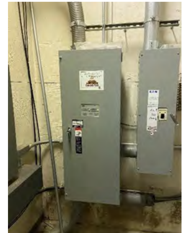
Automatic Transfer Switch
