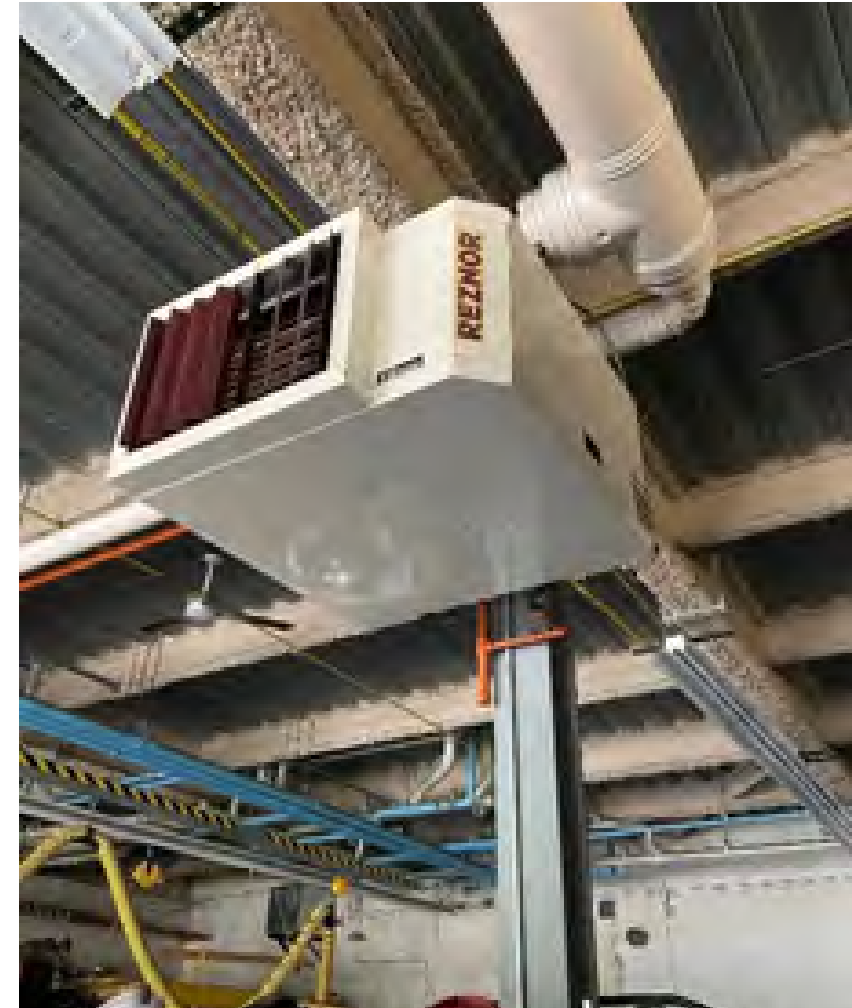
Gas Fired Unit Furnace
