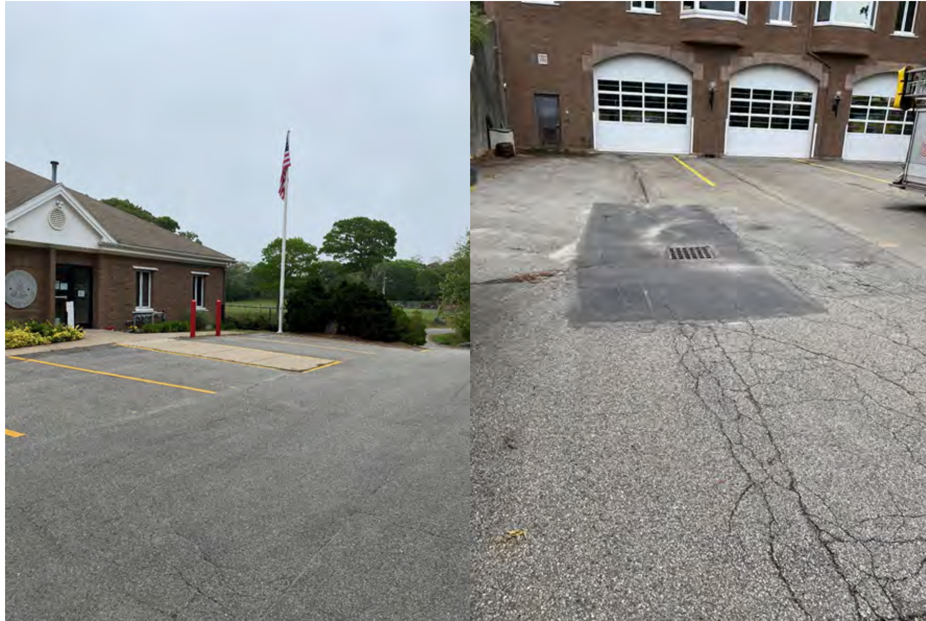
Figure 6: Existing asphalt conditions - Public entrance (left); Lower Apparatus Bays (right). Varying levels of pavement deterioration.
