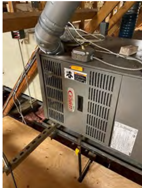
Furnace Unit in Attic Space
