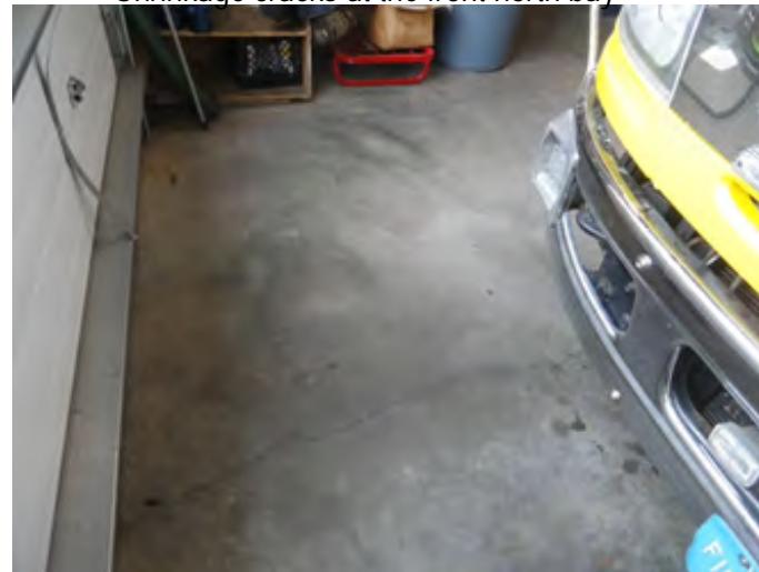
Photo #12 Basement Apparatus Room slab Shrinkage cracks at the front south bay
