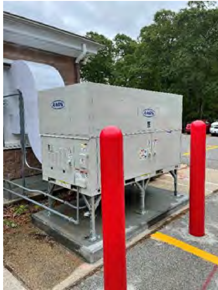
Outdoor Energy Recovery Ventilator (ERV)
