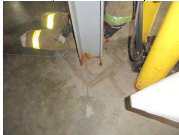
Photo #14 Basement Apparatus Room Surface rust is observed at the bottom of the steel column
