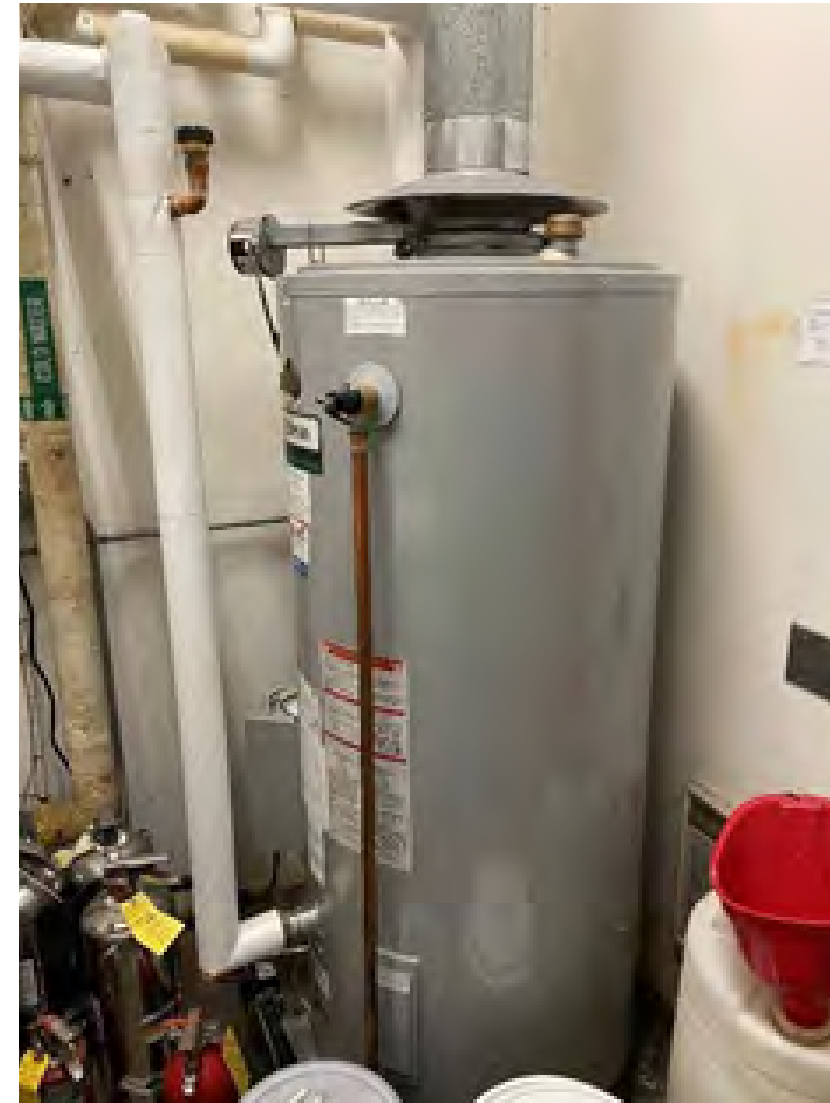
Gas Fired Water Heater
