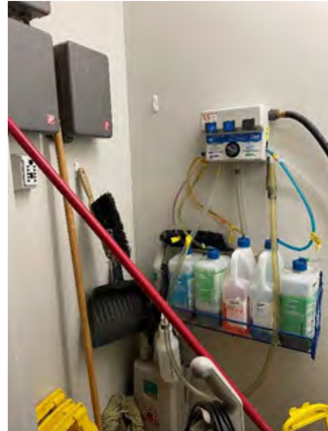
Chemical Dispensing Unit
