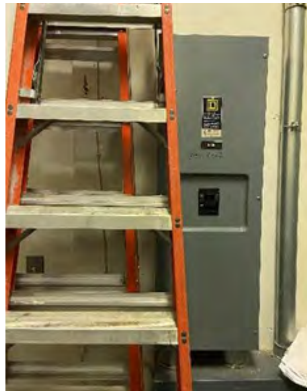
Electrical Service Equipment
