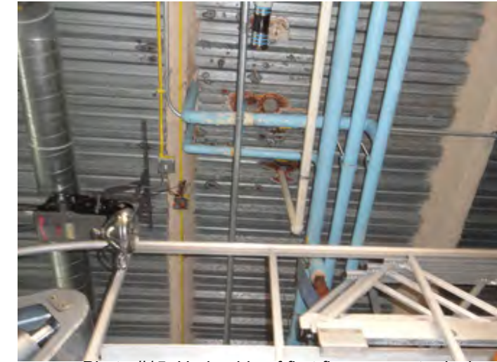
Photo #15 Underside of first floor concrete deck above the apparatus front north bay Surface rust is observed at the steel deck and floor penetrations
