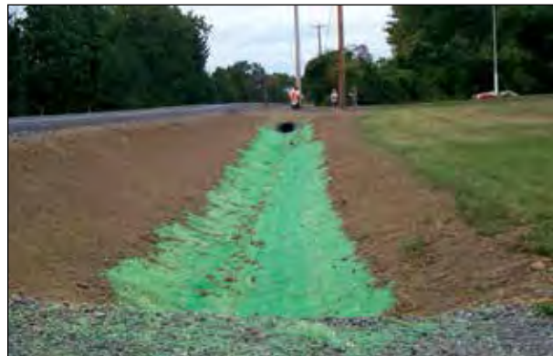
Figure 4j. Erosion control matting can withstand higher velocities of water than most hydraulic mulches.
