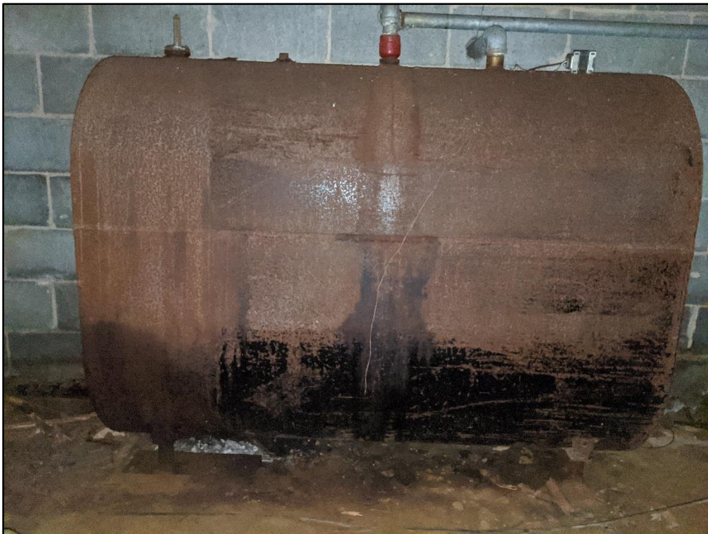
Abandoned fuel oil AST, with soil staining beneath, located in the basement of the Woods View building.
