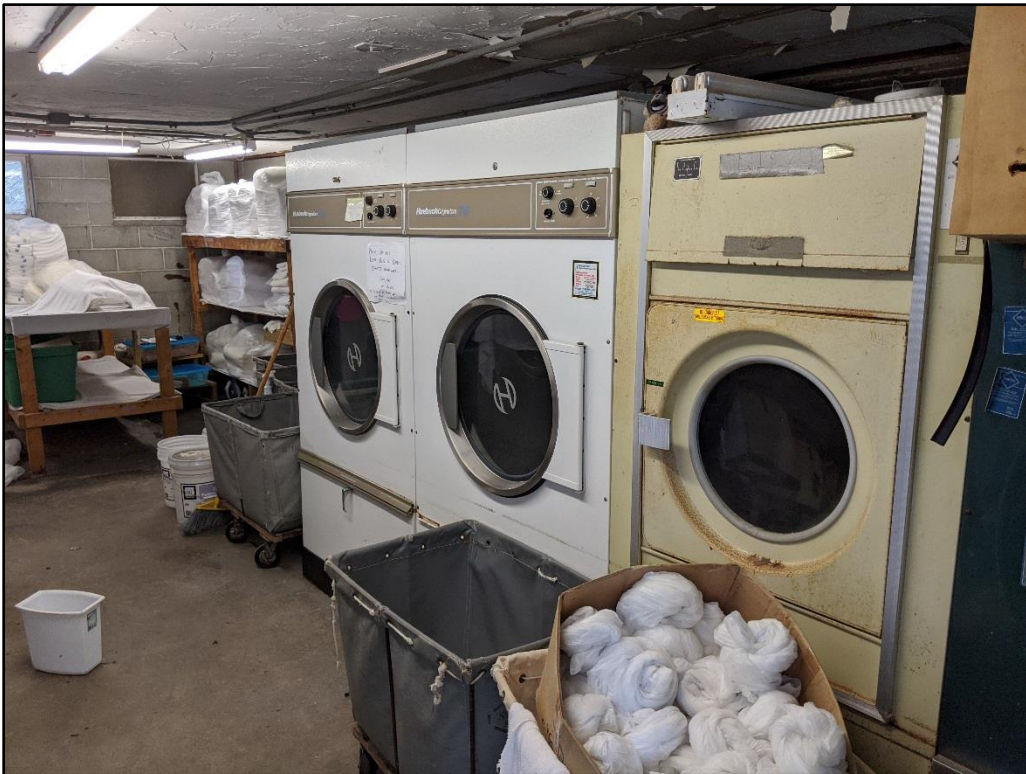
Equipment located in the laundry room, in the basement of the Courtyard 1 building.
