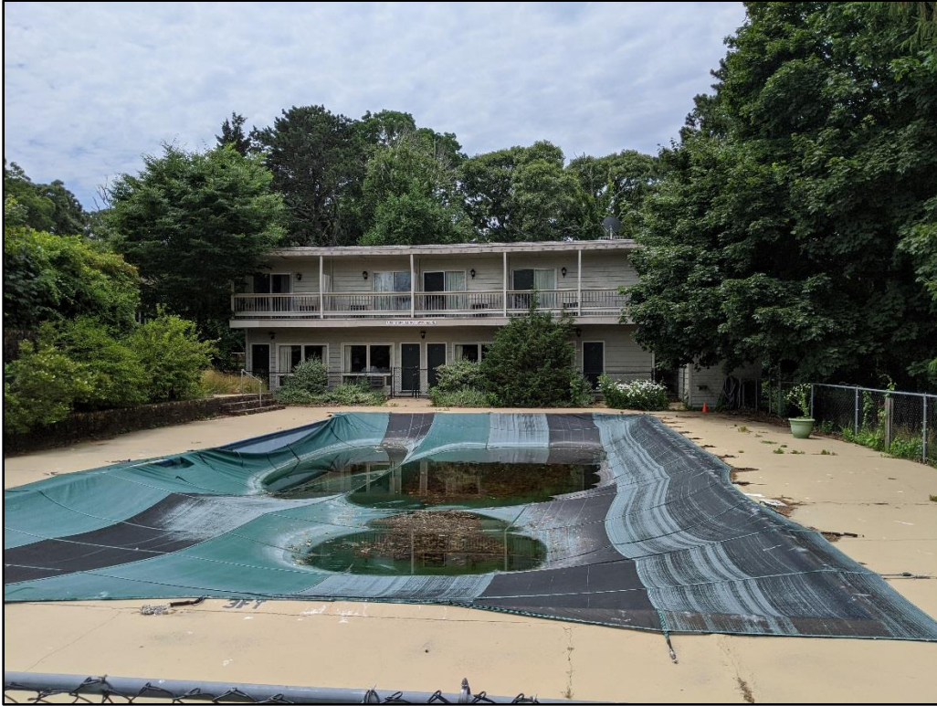
In-ground swimming pool with Pool Building in the background, view facing west.
