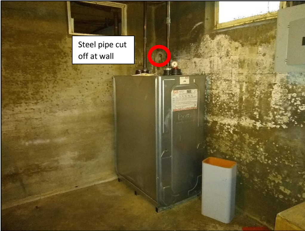
Double-walled fuel-oil AST in the northwest corner of the basement of the building at the 76 Rt 6A property.
