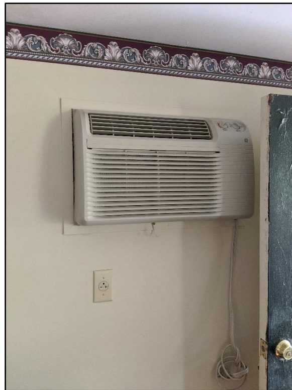
Typical electrical heating/cooling unit found in motel room.
