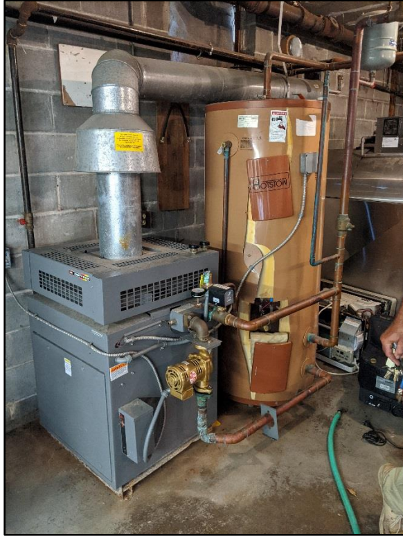
Gas-fired hot-water heater in the laundry room.
