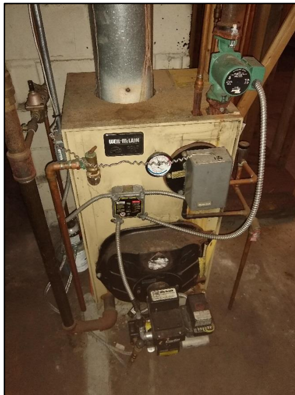
Oil-fired burner in basement of the building at the 76 Rt 6A property.
