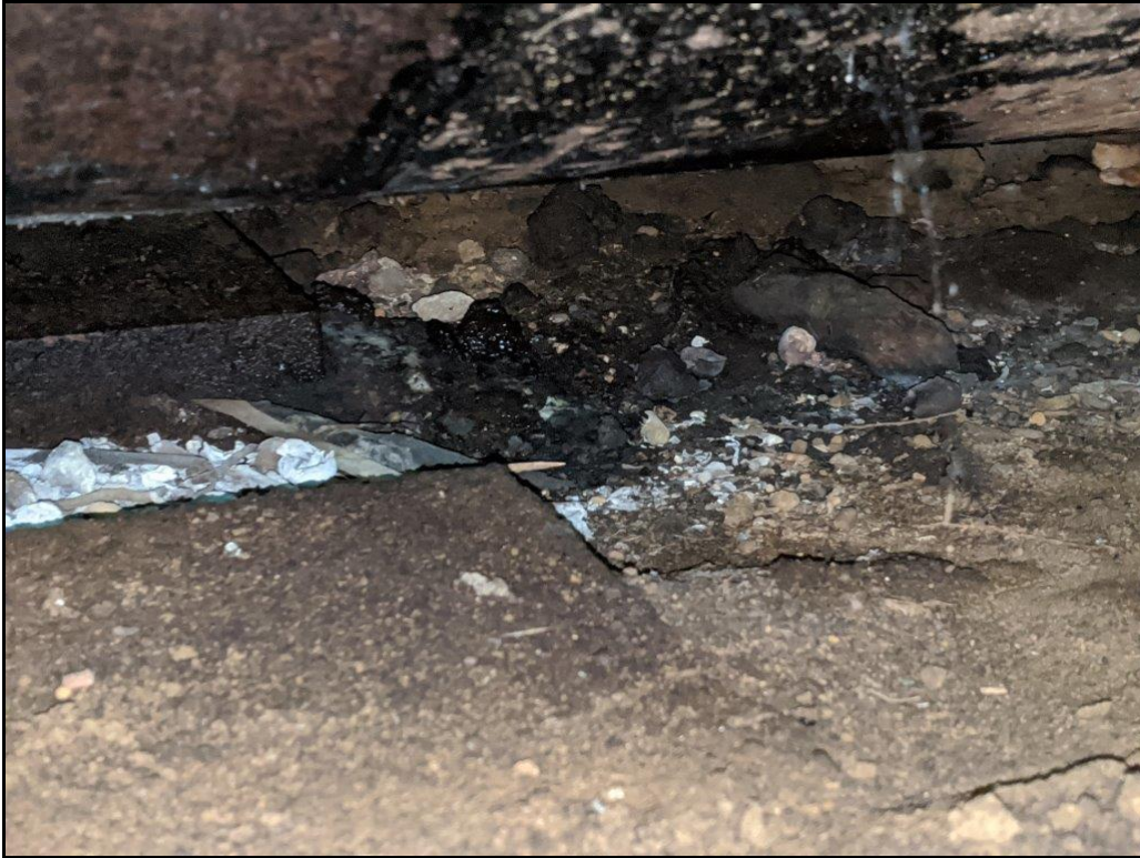
Soil staining beneath abandoned fuel oil AST in basement of Woods View building.
