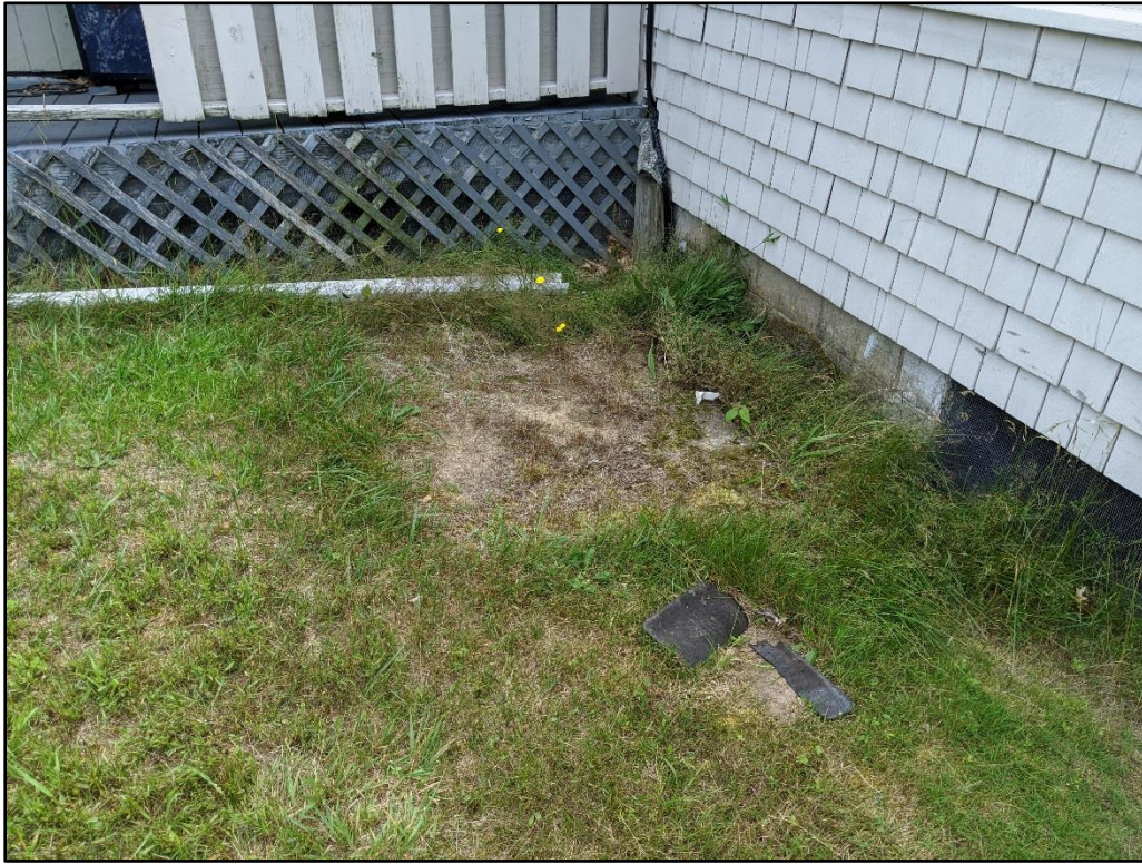
Concrete pad associated with former fuel oil AST, located behind Main Motel Building.
