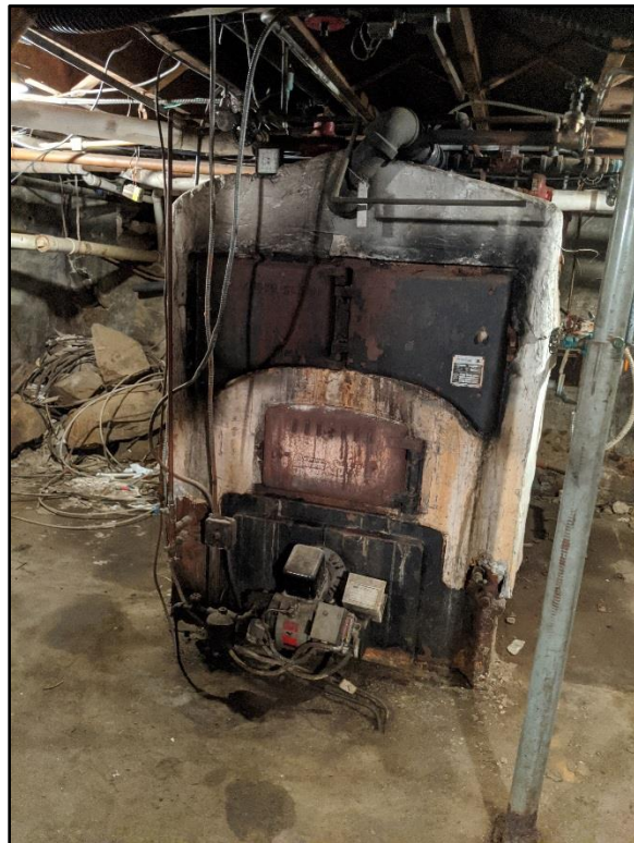
Oil-fired boiler in basement of Main Motel Building.
