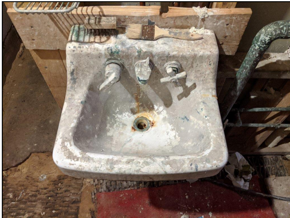
Utility sink with heavy paint staining in the maintenance area in eastern wing of main motel building.
