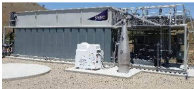
Figure 3-1 Single Train MBR Treatment Module
